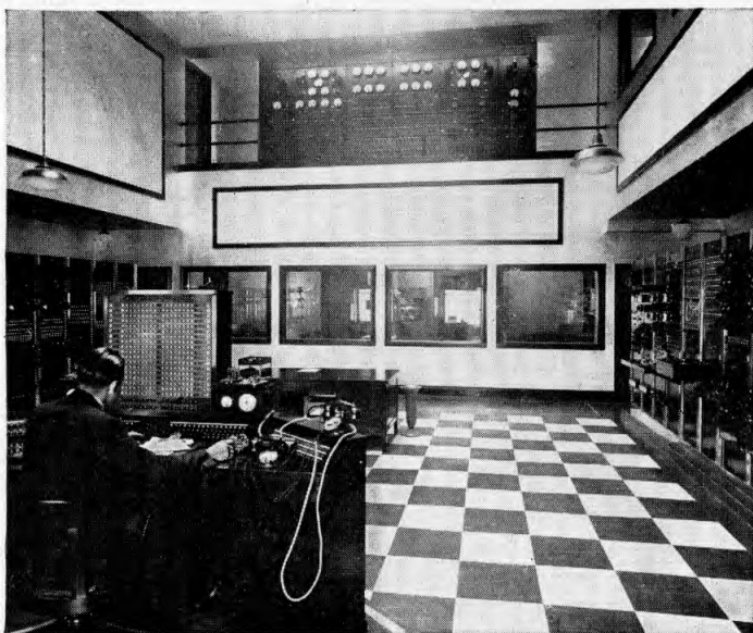
+ The Main Control Room of the N. B. C. studios in Chicago. Here the myriad threads of a nation-wide system of land-wires are gathered together and re-directed into radio channels.
